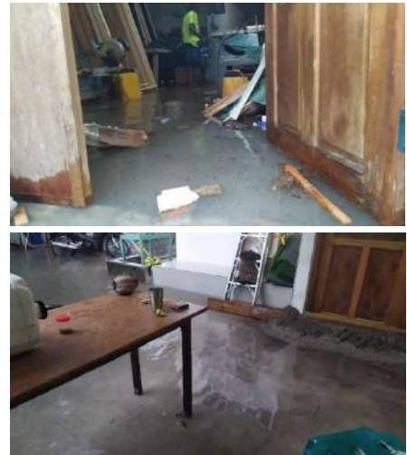
Figure 14: Floods in N. Maalhendhoo on 8 th May.
