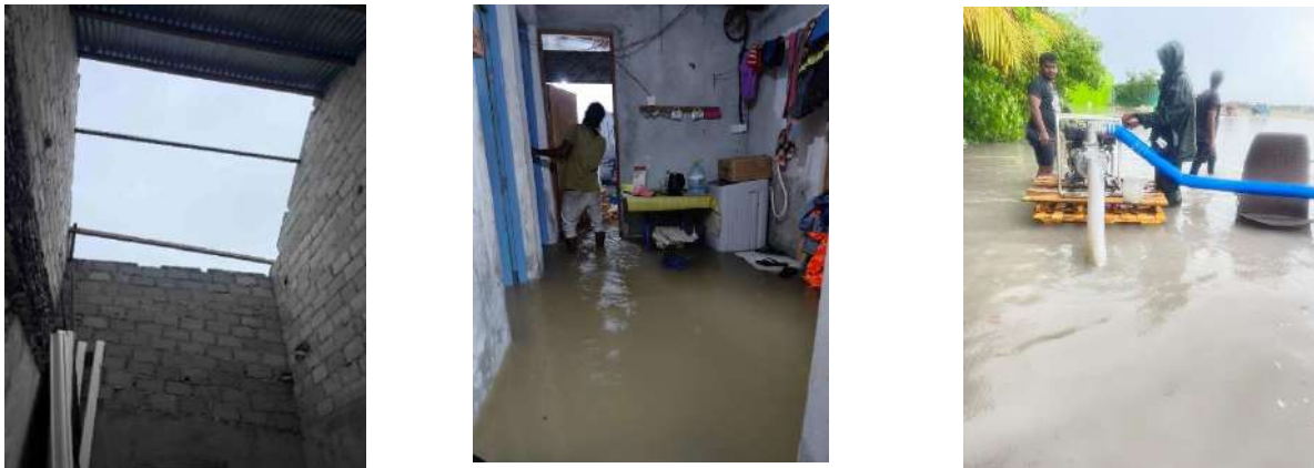
Figure 41: (left) roof damage to a household in Dh. Bandidhoo, (mid – right) Flood waters throughout Lh. Kurendhoo
