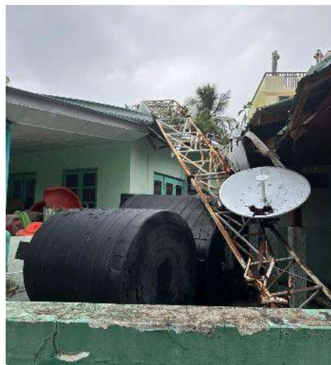
Figure 17: Damage to V. Fulidhoo Council due to strong winds on 19 th May 2024.
