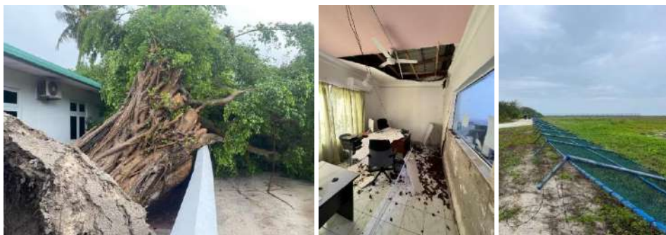
Figure 18: [Left to right] Wind damage incidents from at Sh. Maaungoodhoo health center (21 st May), K. Dhiffushi (23 rd May) and Sh. Funadhoo airport (24 th May)
