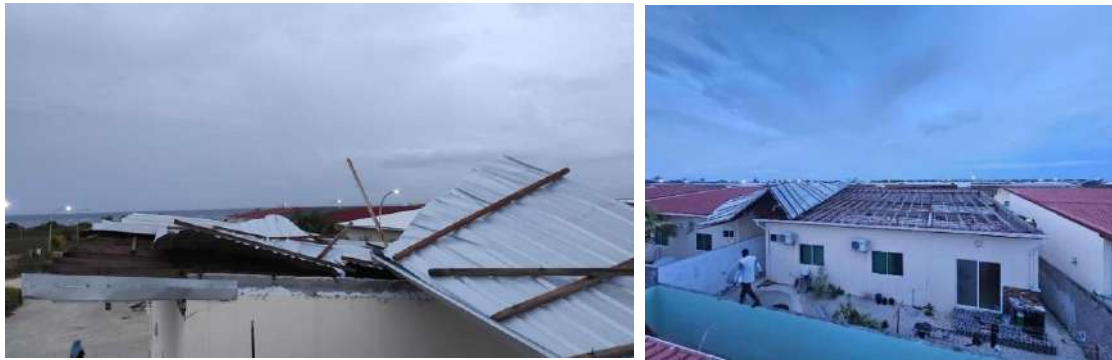
Figure 15: Roof damage in Ha. Dhidhoo on 13 th May 2024.
